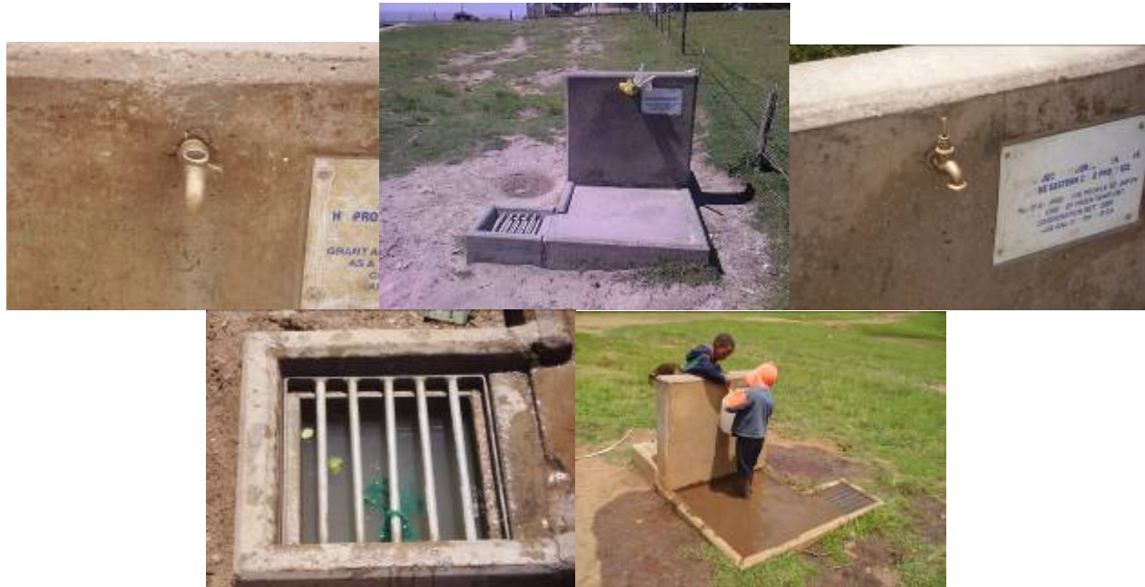
PICTURE 8-12 MAINTENANCE OF COMMUNAL STANDPIPES
