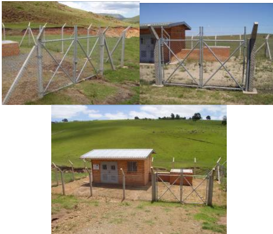
PICTURES 48-50 GATES IN WORKING ORDER
