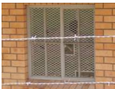
PICTURES 60 VANDALISM AT PUMP HOUSES
