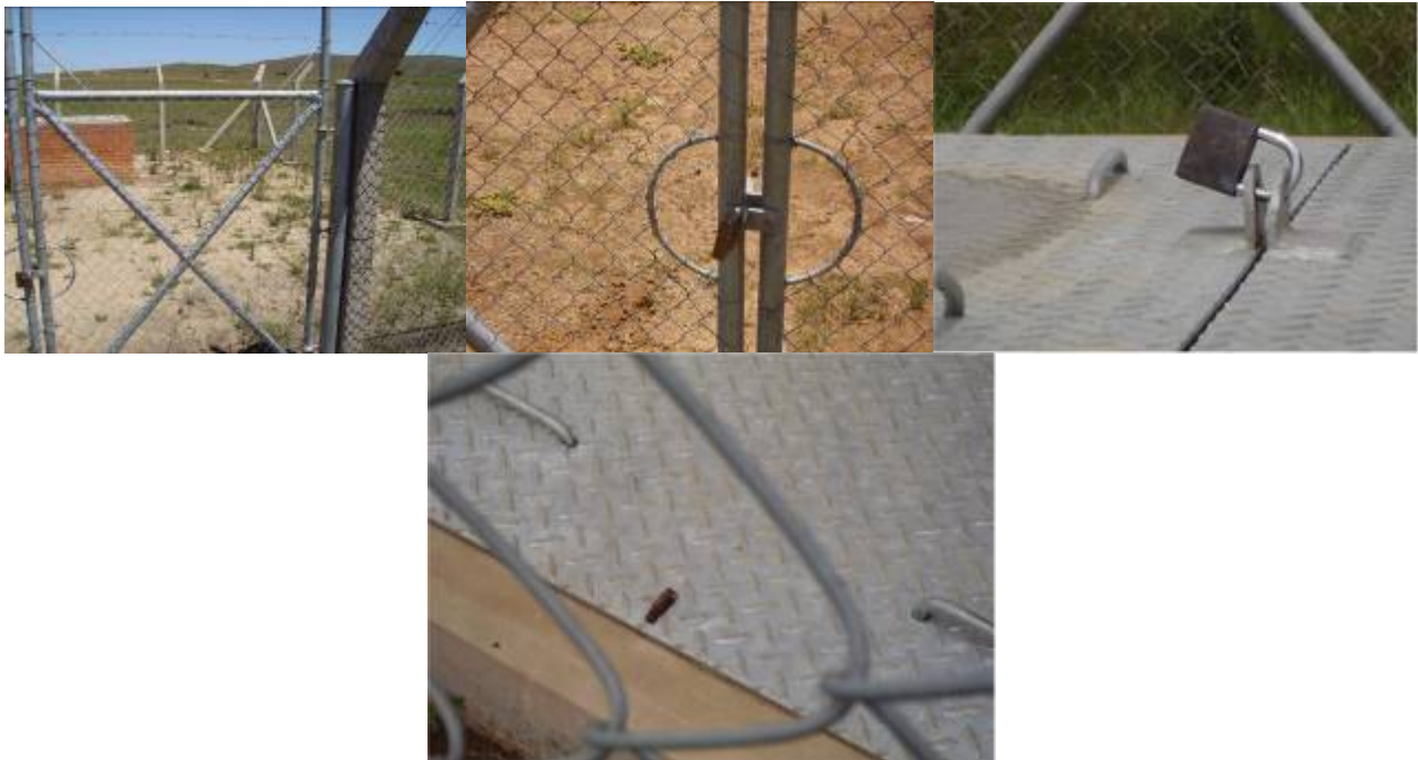
PICTURES 56-59 PADLOCKS IN PLACE
