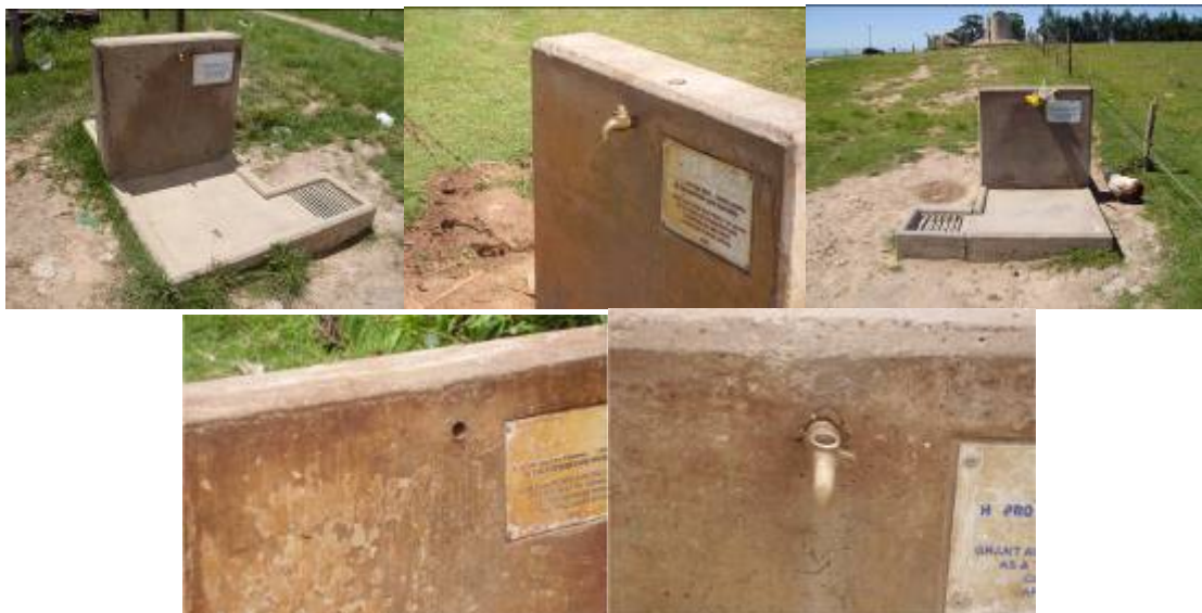
PICTURE 38-42 BROKEN TAPSTAND MECHANISMS
