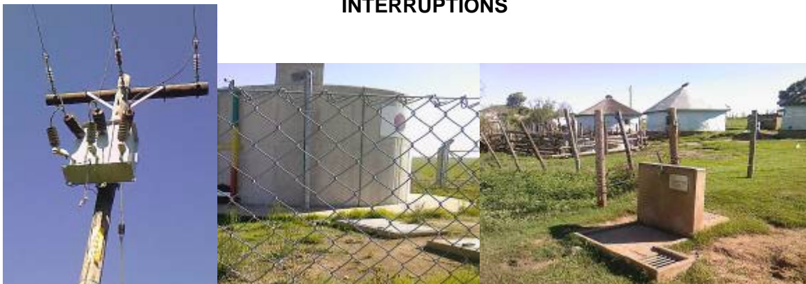
PICTURE 13-15 ELECTRICAL MAINTENANCE WORK AT GUBEVU PUMP HOUSE RESULTING IN WATER INTERRUPTIONS
