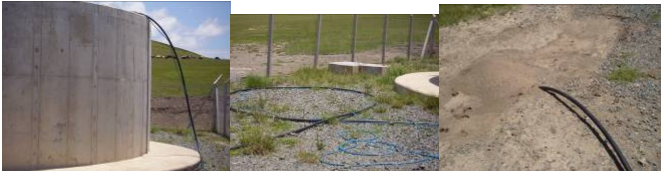
PICTURE 16-18 ILLEGAL CONNECTIONS AT RESERVOIR
