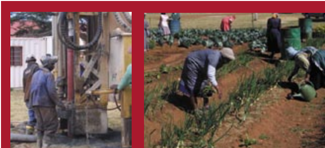
Installation of a bore hole for food garden for an hiv project
